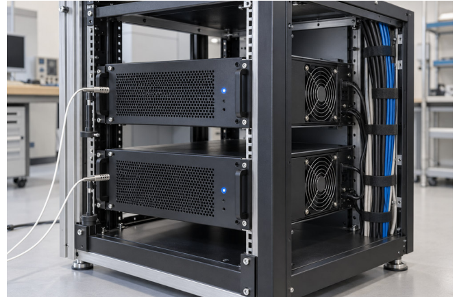
Inlet probes and visible air paths reveal details that a cabinet-average temperature can miss. Generic laboratory rack.
